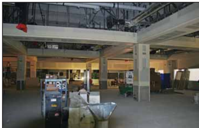
KHS&S craftsmen are completing a wide scope of work in the casino's buffet/kitchen area. Their work includes framing, drywall, painting, millwork and the installation of cultured stone.
